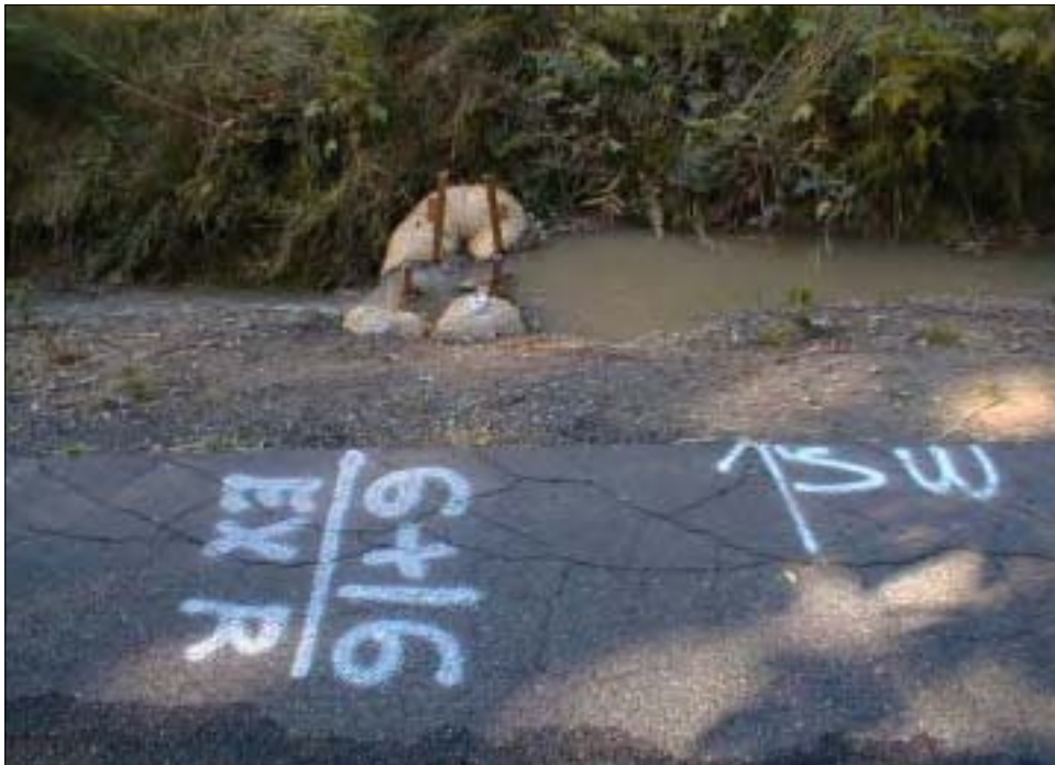
Coir log used to allow settling and to decrease water velocity/erosive forces
