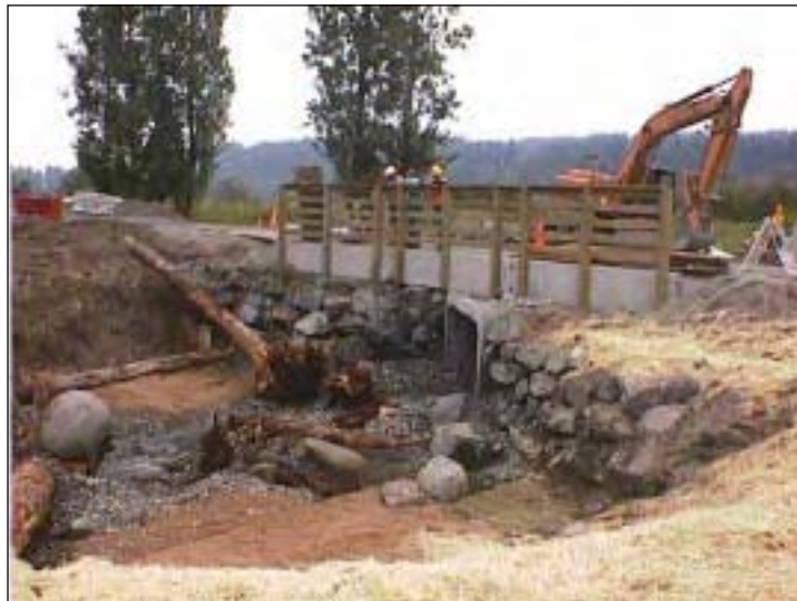
Large woody material placed in streambed to provide fish refuge. Note use of streambed gravel, mulch, and coir fabric
