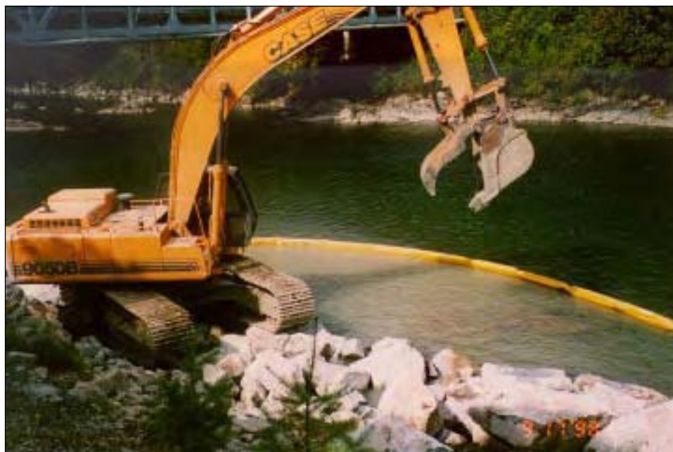
A river repair project in progress using a turbidity curtain to contain turbid water
