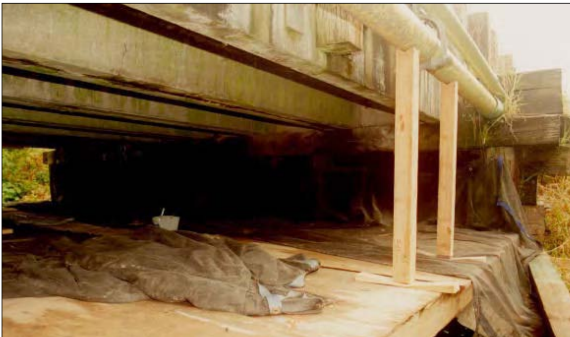
Plywood work platform providing a safe work environment and containing fallen debris from entering water during construction, maintenance, and repair activities
