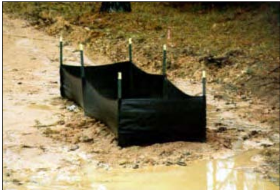
Inlet protection: filter fence surrounding catch basin to reduce soil particles from entering drainage system
