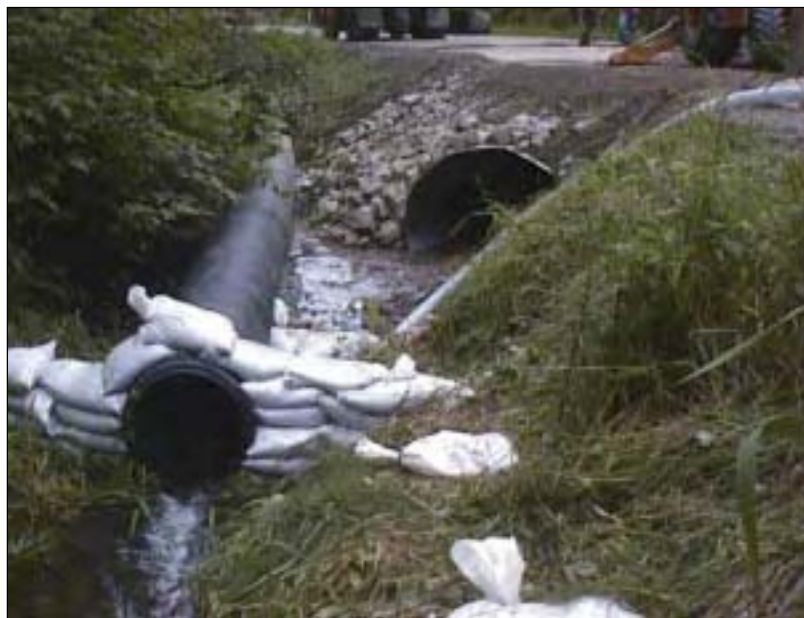
Sandbags holding bypass pipe in place and detaining sediment laden water on site
