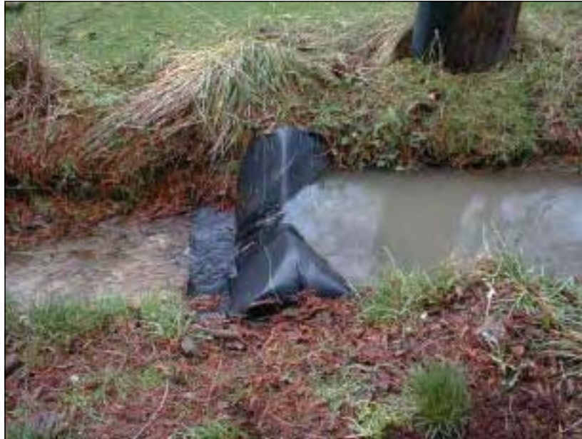
A triangular silt dike detaining water and allowing soil particles to settle
