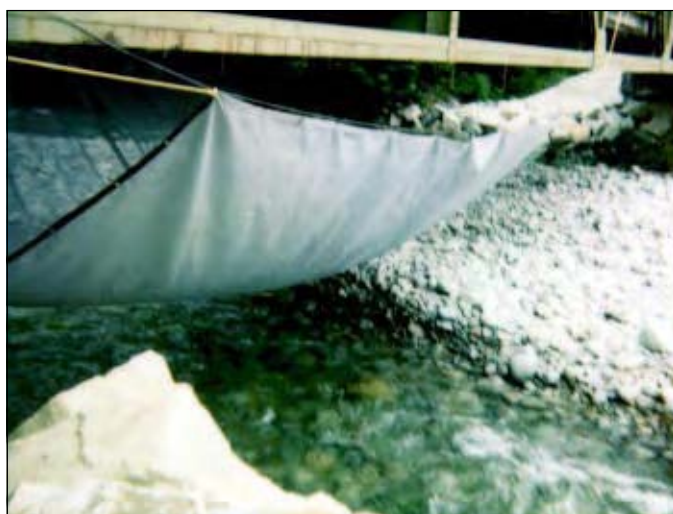
Diaper netting under bridge
