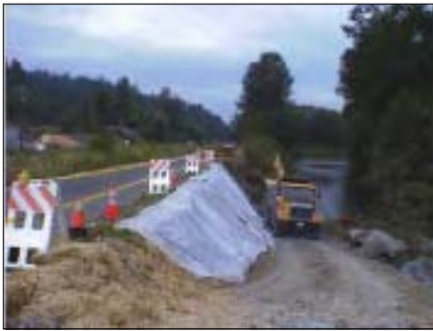
Plastic covering used as erosion protection on a slope at construction/repair area. Note additional use of mulch in area
