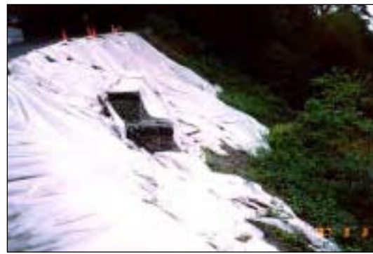
Plastic covering used to protect exposed surface from erosion during construction/repair activities
