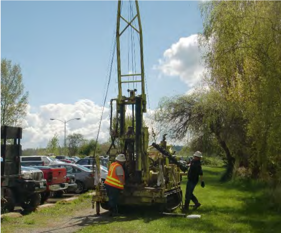
Figure 2-3. Example of a Medium-Sized Track-Mounted Rotary Rig with a Fully Extended Boom. The model in the photograph is a CME-850.
