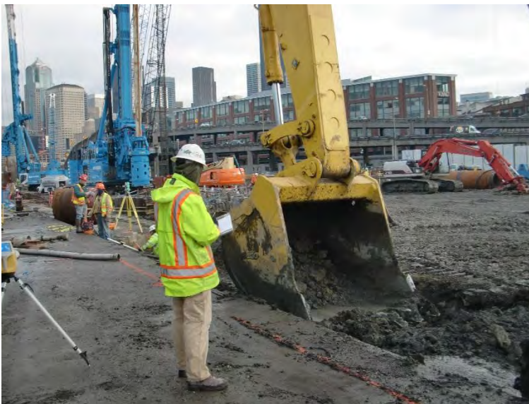
Figure 2-11. Example of Excavation Performed with a General Use Bucket with Teeth. Note that the general use bucket in this photograph is particularly large and attached to a large excavator.
