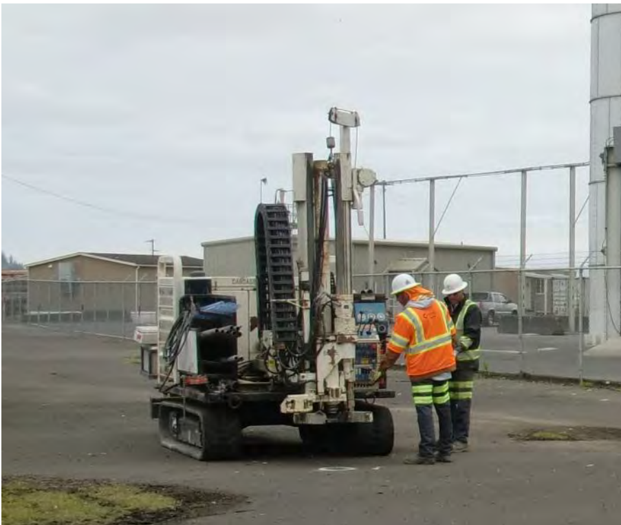
Figure 2-2. Example of a Medium-Sized Track-Mounted Geoprobe Rig (Rinck et al. in press). The model in the photograph is a Geoprobe 7730.
