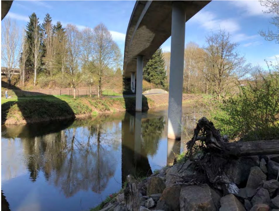
Figure 3. Northbound I-405 to Eastbound SR 522 Ramp with Two Piers Proposed for Removal in the Sammamish River
