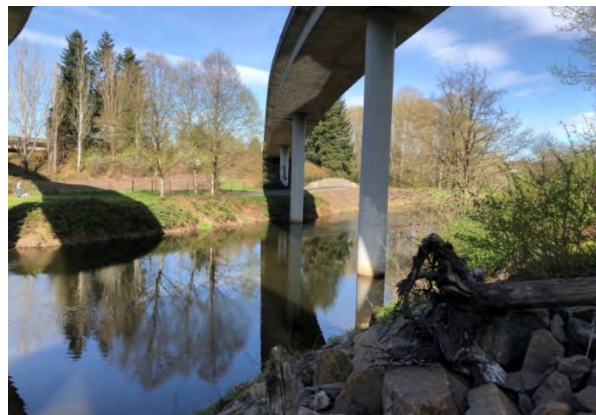
Northbound I-405 to eastbound SR 522 ramp with two piers proposed for removal in the Sammamish River.
